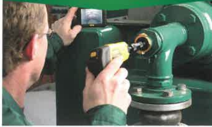
Camera inspection in centrifuges
